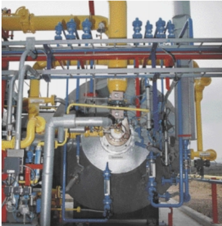
View of a two-stage burner system
