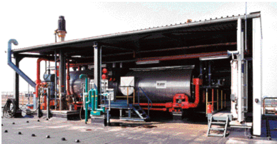
Combustion chamber and steam boiler of a system for oxidation of CHCs
