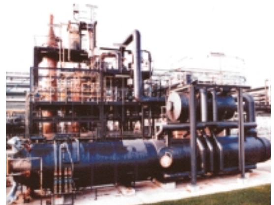
Combustion chamber and fume tube boiler of a CHC oxidiser
