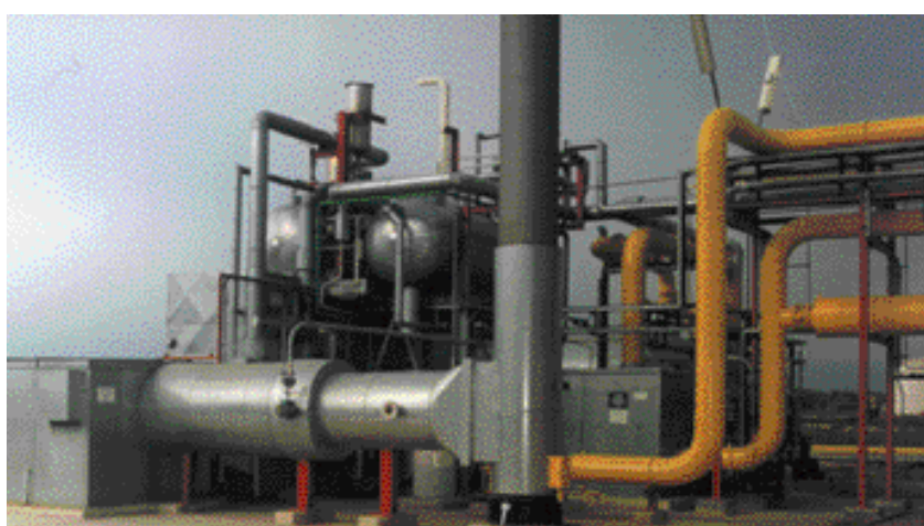
Turnkey system for purification of explosive exhaust gases
